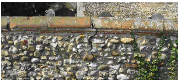
Picture 1.14 Wall surrounding graveyard, small area in need of repair.
