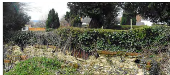
Picture 1.15 Part of boundary wall within graveyard in need of repair.
