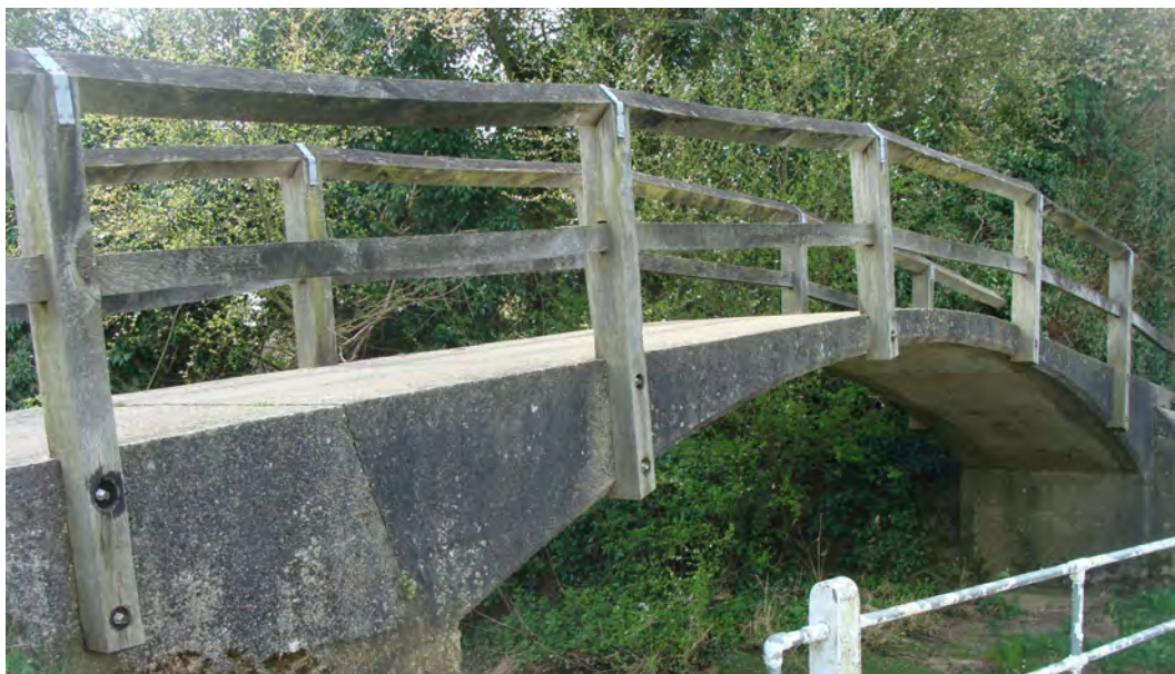
Picture 1.21 Delicately proportioned bridge crossing River Chelmer. It and metal safety railings would benefit from maintenance and repainting.
